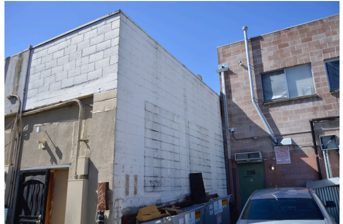
Figure 2. Rear of building viewed from alley. Concrete block and window openings infilled with concrete block are visible at this corner of the building, looking southwest.
